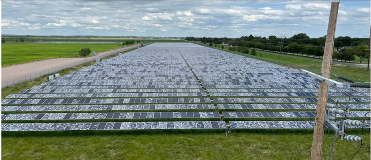
A solar farm near Scottsbluff, Nebraska, suffered major damage in June 2023 when a storm dropped baseball-sized hailstones at 100 to 150 mph on it. (Courtesy Photo)
